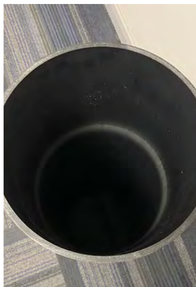
The ducting has a diameter of 225mm
