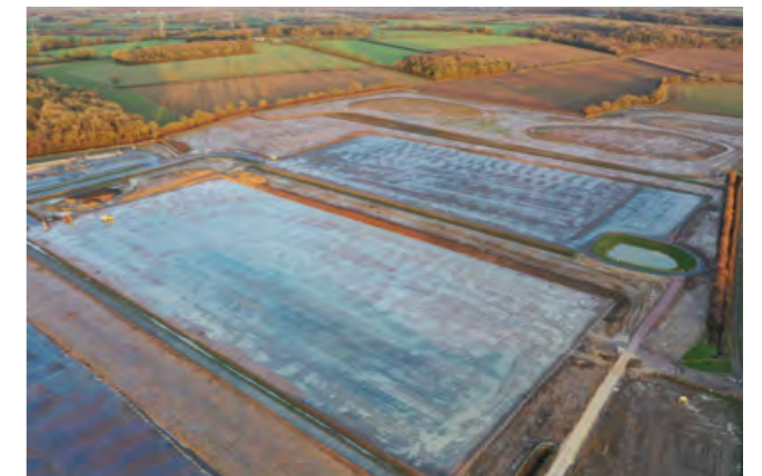
Converter hall platforms
