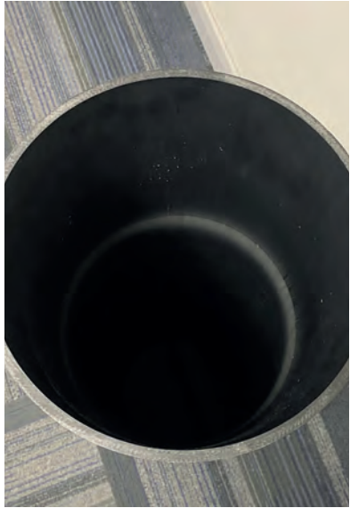
The ducting has a diameter of 225mm
