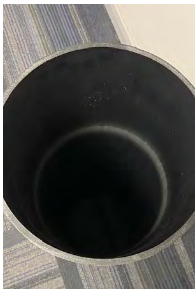
The ducting has a diameter of 225mm
