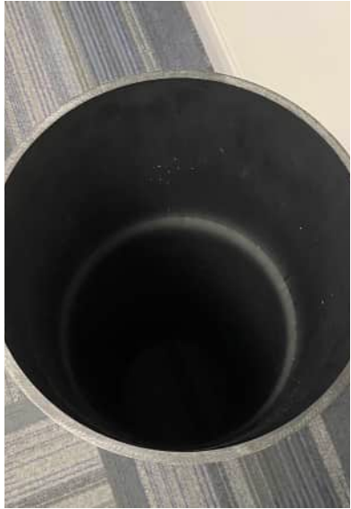
The ducting has a diameter of 225mm
