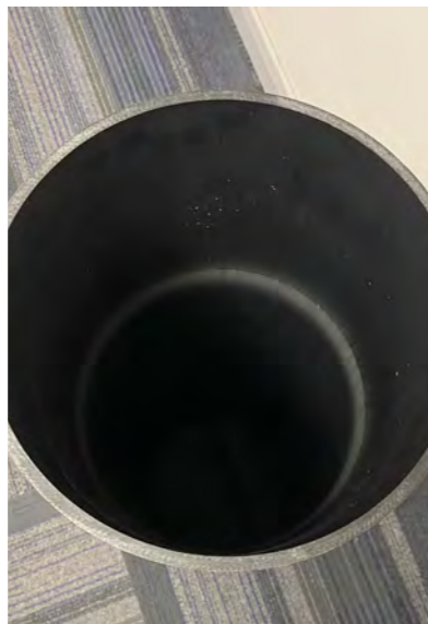
The ducting has a diameter of 225mm
