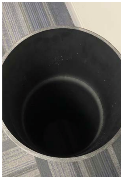
The ducting has a diameter of 225mm
