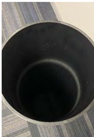
The ducting has a diameter of 225mm
