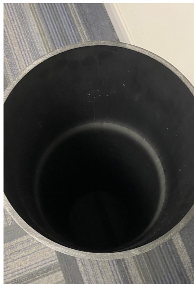
The ducting has a diameter of 225mm
