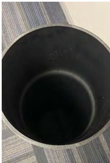
The ducting has a diameter of 225mm
