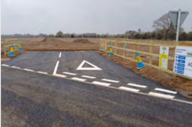
Almost all of the temporary access points (example shown above) have been installed along the cable route. They will be in place until all cables are installed, then removed and land reinstated.
