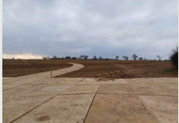
The weather over the winter months was not ideal for mainline ducting but the Murphy team continued work on Horizontal Directional Drills. The laydown area for an HDD is pictured above. You can read more about this process on page 8.
